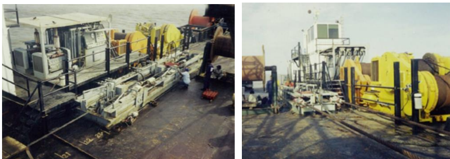
Linear pull winch arrangement on a floating barge anchored 4.5km off landfall and 500m from inter-tidal zone
