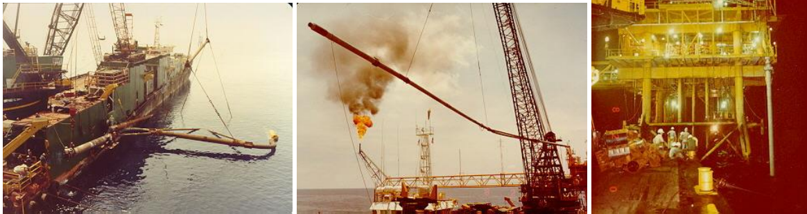
After installing the U-bend, the riser was added and the assembly lowered to seabed with riser installed inside riser clamps
