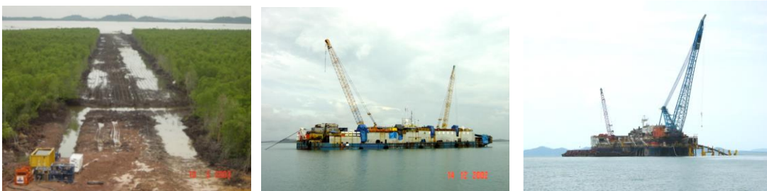
(Left) Reinstatement of site including mangrove planting; and (Right) two laybarges used for installing the long pipeline
