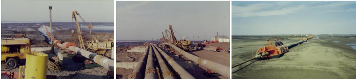
Pulling of pipe strings with buoyancy tanks from onshore stringing yard to pull barge location
