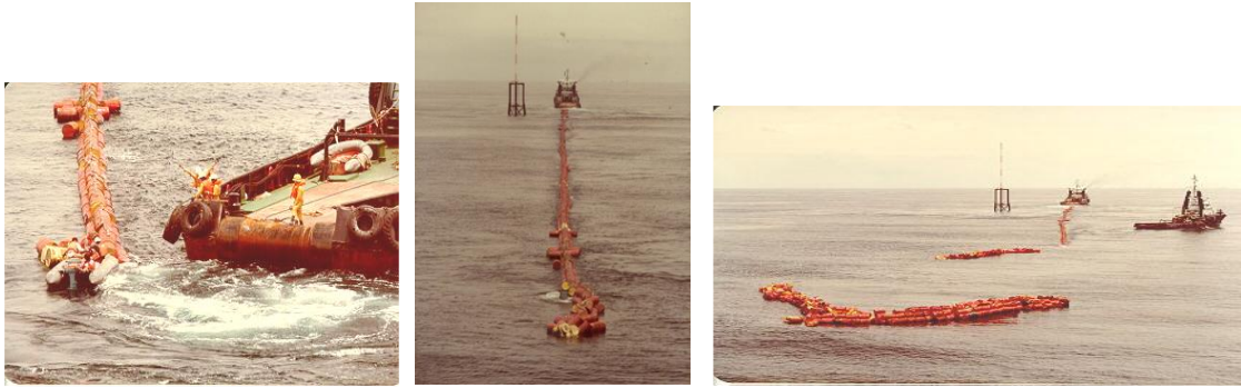
Stripping of buoyancy drums from pipeline while applying tension to lay it down to seabed
