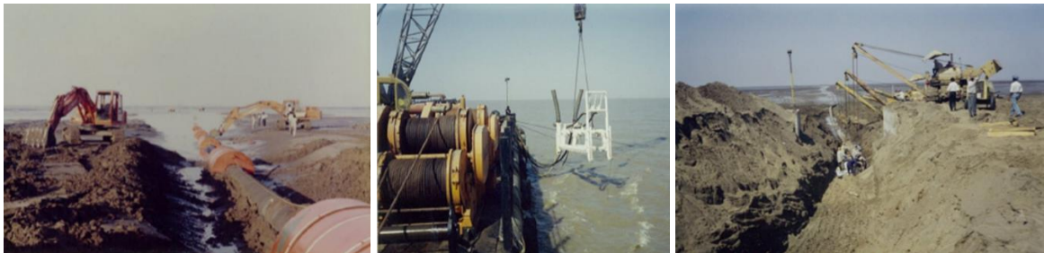
Burial of subsea pipeline via jet sled (offshore) and excavator for inter-tidal zone and onshore
