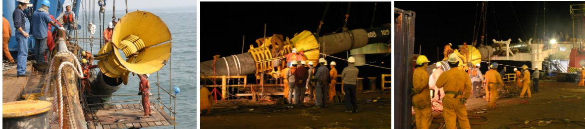
Installing Stabbing Guide to facilitate Alignment & Welding of PLEM spool to Pipeline
