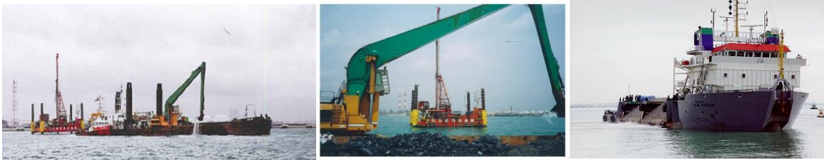
(Left & Middle) Simultaneous dredging and drilling & blasting works for trench preparation & (Right) side-stone dumping vessel for backfill installation
