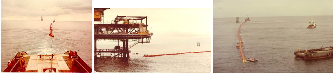
Towing of pipeline bundle to offshore platform, tying to initiation cable and retrieving stripping wire from bundle
