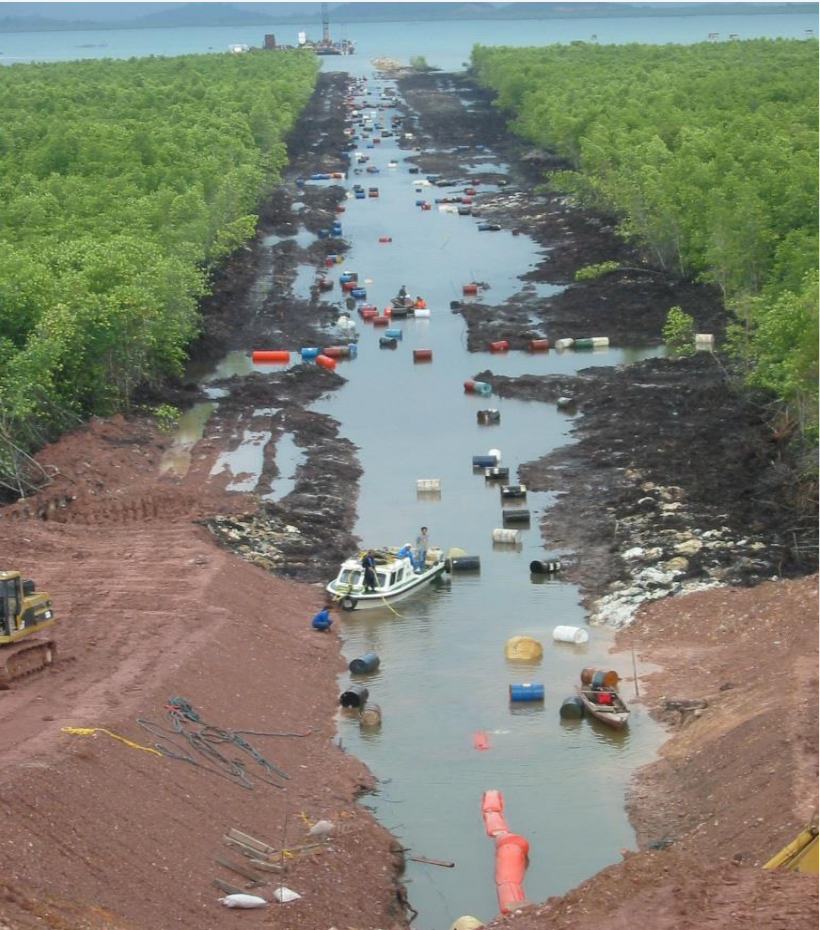
Collection of oil drums after being stripped from pipeline to allow it to settle onto Seabed
