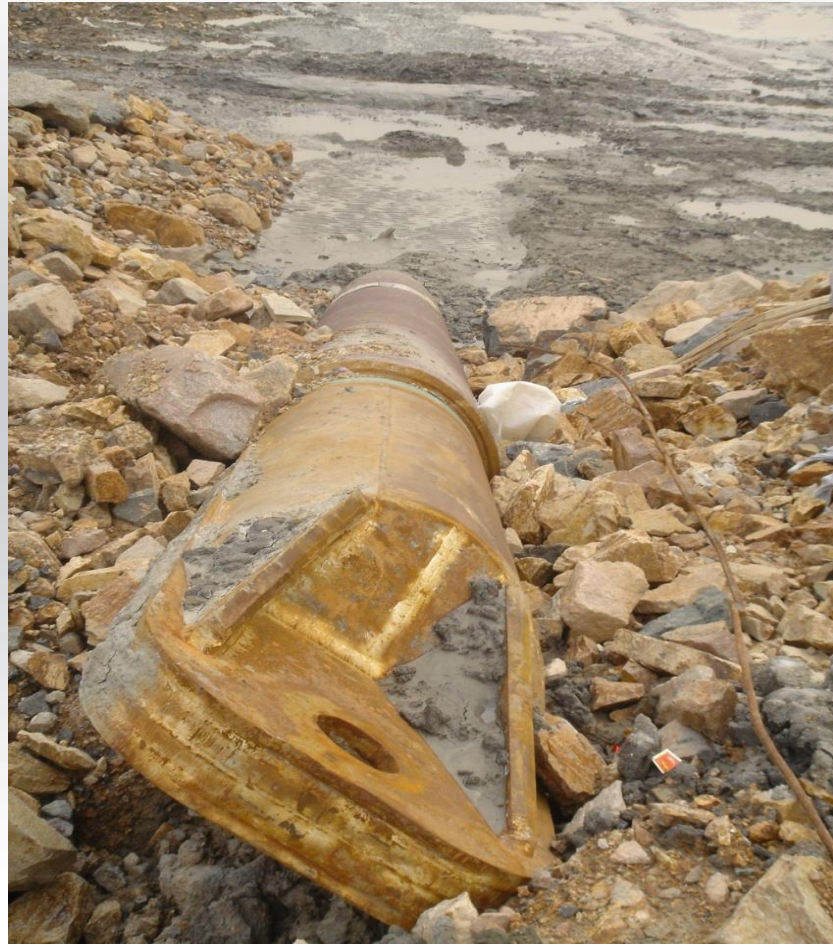
Pipeline pulling head at the HDD entry point and all HDD equipment removed
