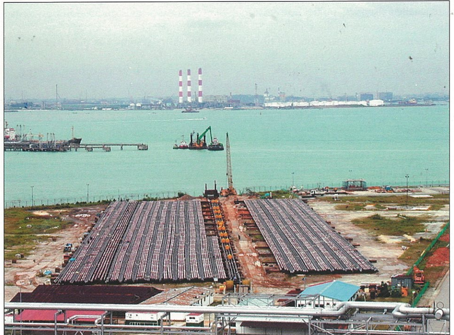
The stringing yard on Pulau Ular (the launch site; see Fig. 1) looks across the Sinki Fairway at Jurong Island (the landing site; Fig. 2). Photograph from Kvaerner E&C, Singapore.
