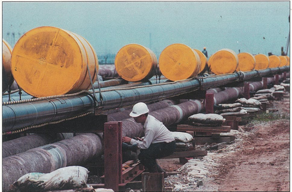
Kvaerner project manager Ng Eng Bin inspects pipeline bundle with buoyancy tanks in place just before installation begins (Fig. 7). Photograph from Kvaerner E&C, Singapore.
