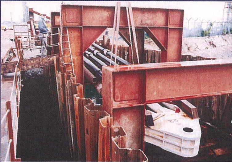
The end of the pipeline comes into view between the sheet piles at the shore approach.
