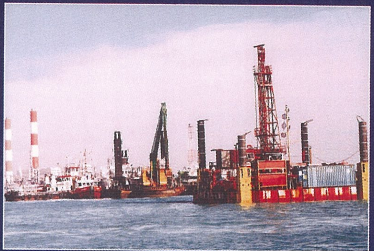
624 linear m of trench required blasting, which was performed by two separate spreads and then excavated by the Ave Caesar .
