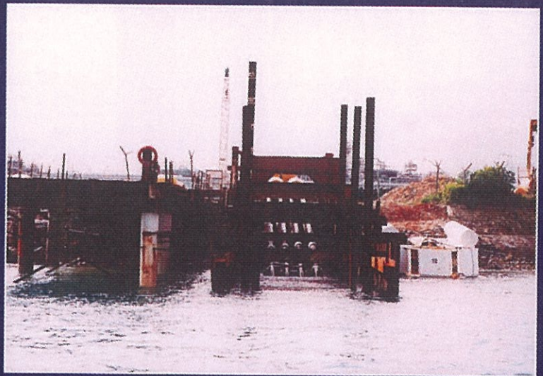
The pipeline shore approach at Pulau Ular, where the bundle can be seen on the launchway rollers inside the cofferdam.
