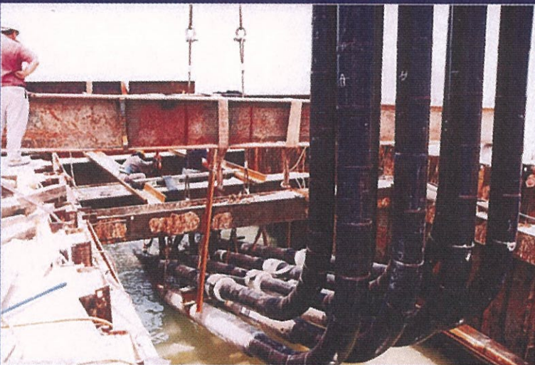
Space limitation required a riser to be installed at each end of the pipeline to bring the tie-in points as close as possible to the shore line.
